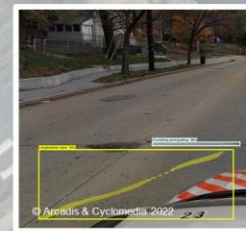
CONCRETE DEFECTS COMPUTER VISION
