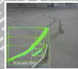
WAREHOUSE DEFECTS COMPUTER VISION
